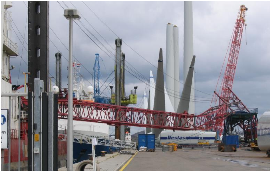
A crane collapsed in the marshalling harbour
