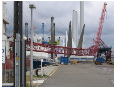
A crane collapsed in the marshalling harbor
